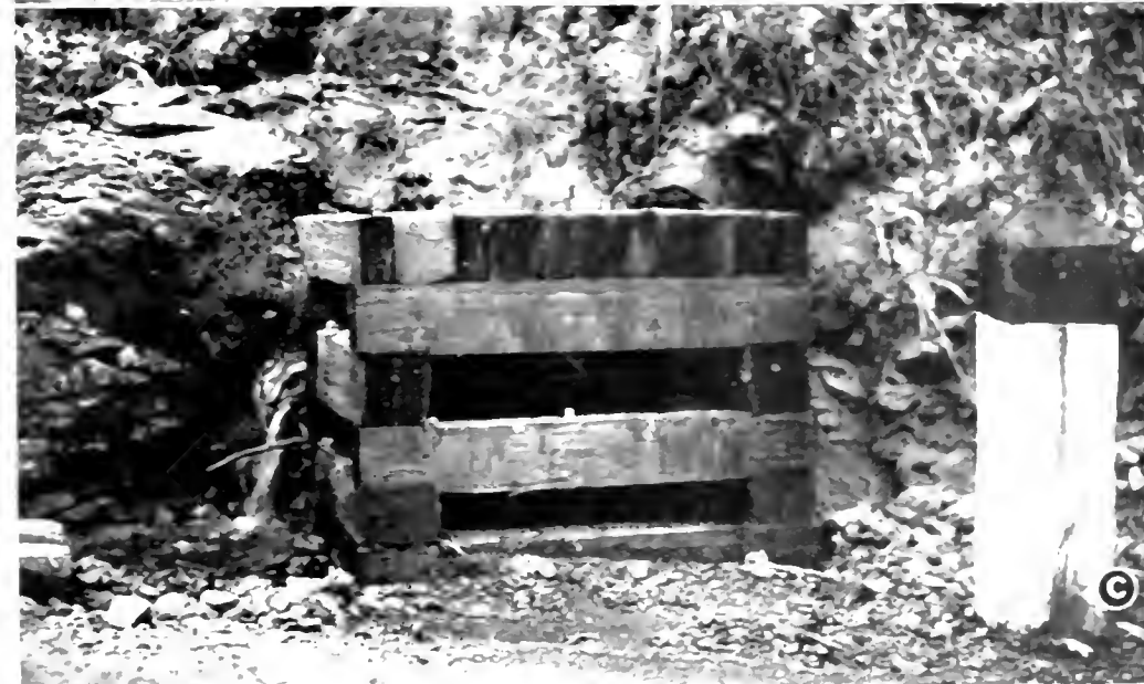
FIGURE 10. a) Debris crib of reinforced concrete, with provision for extension placed over culvert entrance in small debris basin and commonly known as a "bear trap." b) Timber debris crib installed over culvert entrance in roadway gutter. Note how debris has been prevented from blocking culvert entrance. c) Debris crib of new timber, with a solid cover, placed over culvert entrance in roadway gutter.
